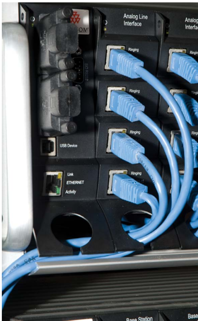
Figure 1-9 Harnessing cables to the side and out.
