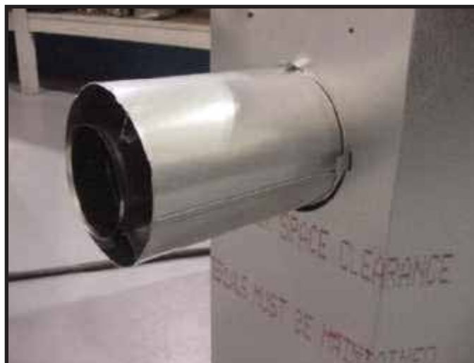
Figure 9.10 Attach the first vent section (it will snap into place). Slide the insulation gasket onto the vent section, up against the appliance and over the tabs.
